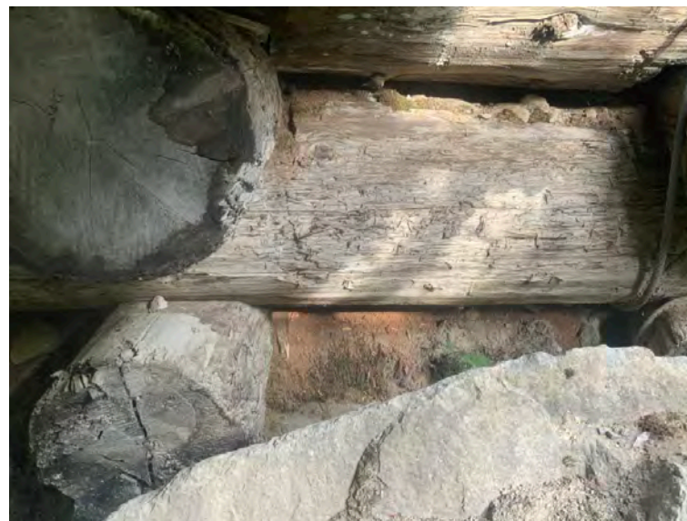
Left Bank Abutment when facing downstream, saw dust.
